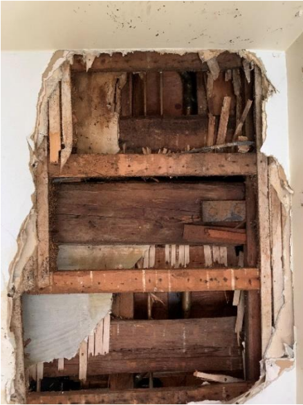
18 th century plaster and lathe are visible next to the large wood beam at the center of this photograph.
