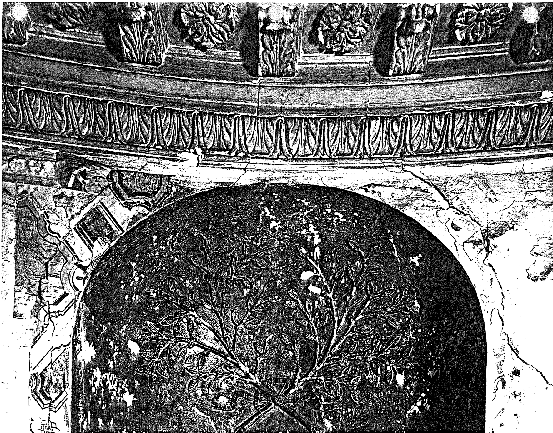
Fig. E-15. Shirley-Eustis House, Roxbury, Ma. East Hall detail of ornamental plaster in niche on west wall and ornamental plaster cornice. Compare detail of cornice to Daniel Raynerd (Bulfinch's plasterer) designs for "Fancy Cornices" (Fig. F-19). J. David Bohl photo, August, 1979. (SPNEA)
