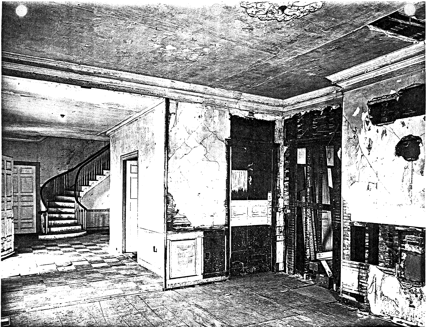
Fig. E-7. Shirley-Eustis House, Roxbury, Ma. Southwest Breakfast Room looking northeast showing Georgian floor, dado, door, wood cornice; Federal plaster patch above dado; Victorian plaster cornice and chimney breast; Modern removal of original partition. J. David Bohl photo, August, 1979. (SPNEA)
